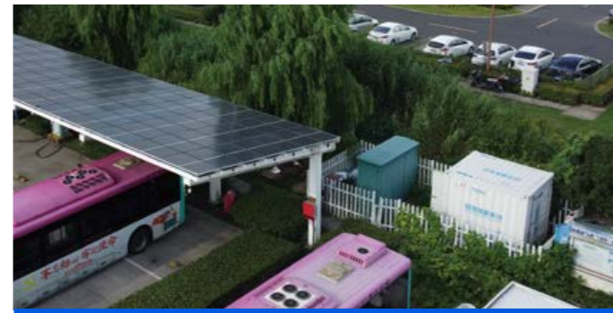
Tongli Bus Station PV-Storage-Charging Project
