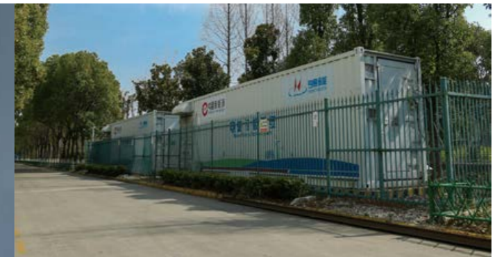
Cable Factory Containerized Energy Storage Project
