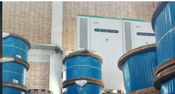
PV & Energy Storage Project
