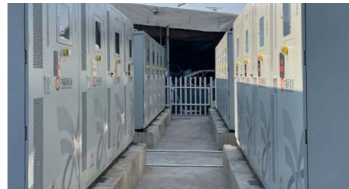
Limin C&I Energy Storage Project
