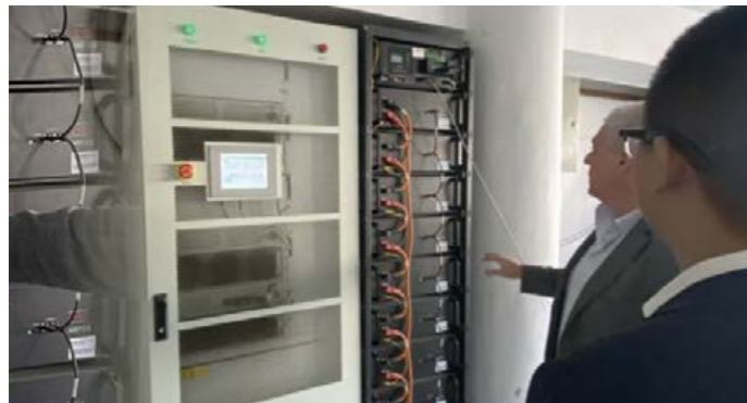
C&I Energy Storage Project
