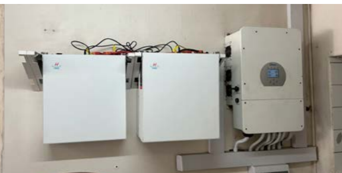
Residential Energy Storage Projects
